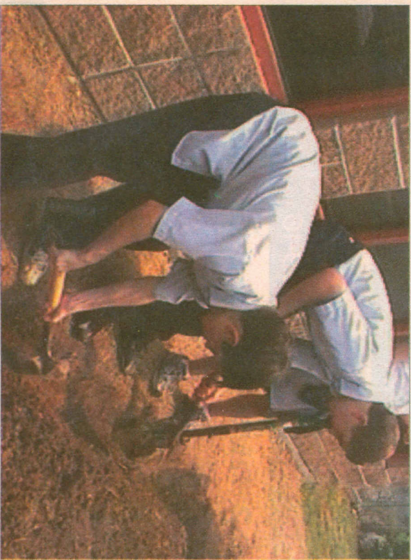
Our Lady of Mercy students Patrick Talbot and Drew Maranto pitch in to help with digging for the nursery and automated sprinkler system. Photo provided by Our Lady of Mercy School
